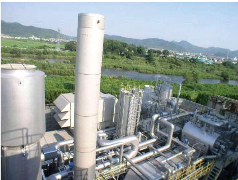
Photo: Cogeneration Facilities at the Himeji Factory
