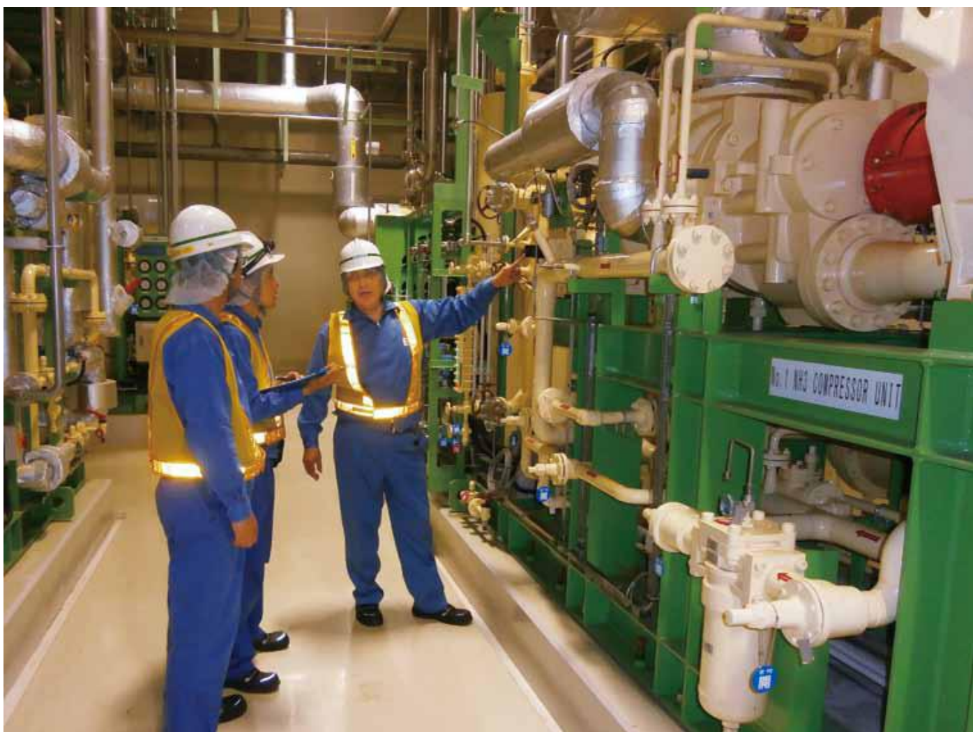
Non-Freon (CO 2 /NH 3 ) Cascade Refrigeration System (Shimada Factory)
